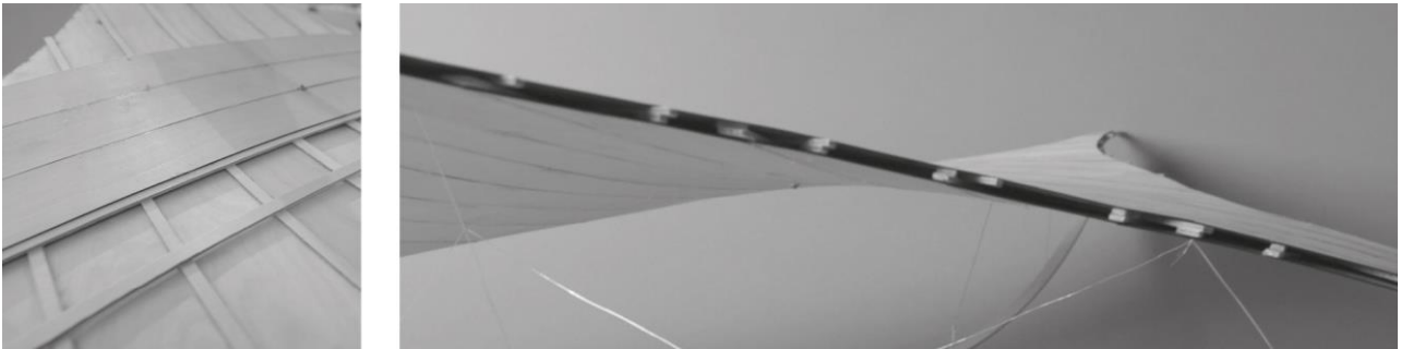
Figure 12: Fixing the second wooden-surface onto the structure providing a self-formed composite shell
